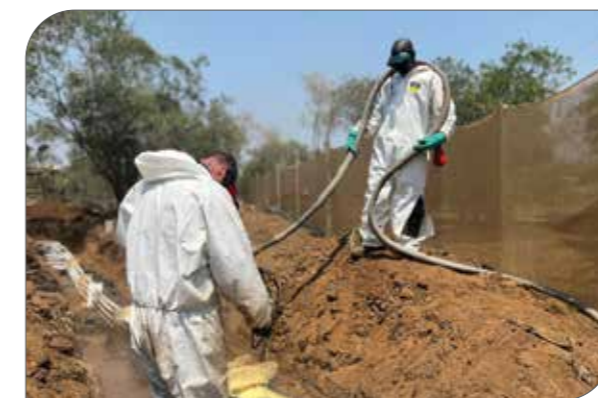
Before and after of foaming trenches to insulate piping to Monwana Spa, by Reliance Foam. The foam gun sprays a mixture of isocyanate and resin through a heated gum. The mixture solidifies and expands on contact.
