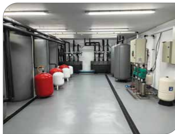
Boilernova hot water buffer tanks, expansion vessels and distribution stations.
