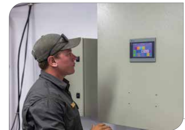
Colin Holden from Monwana viewing the PLC control system home screen.
