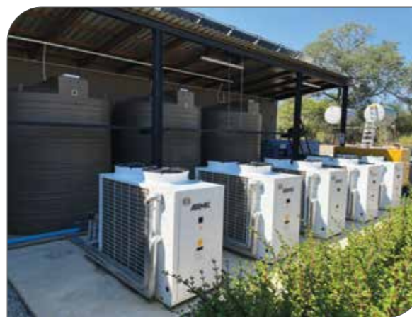
ANL desuper heat recovery units.
