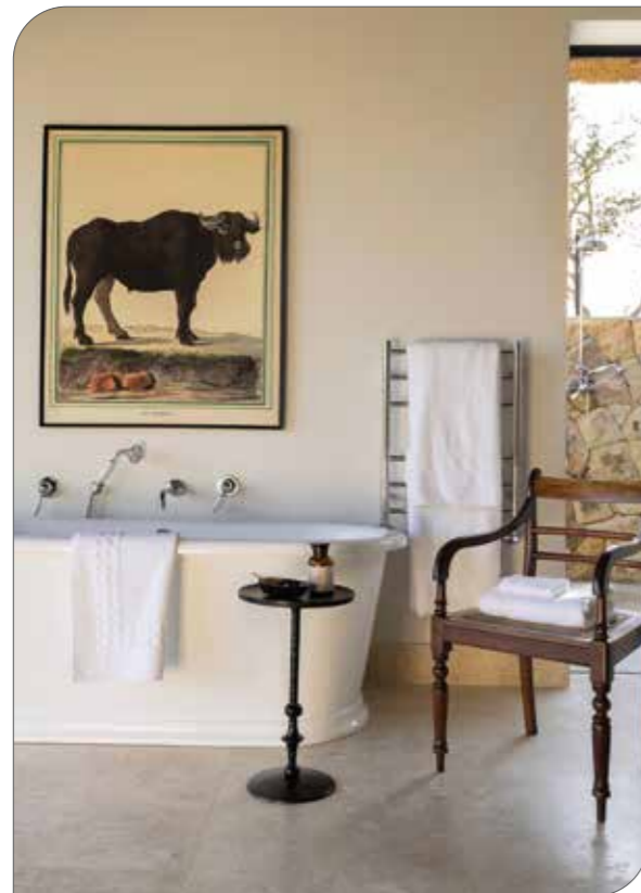
Bathroom with underfloor heating and hydronic heated towel rails.
