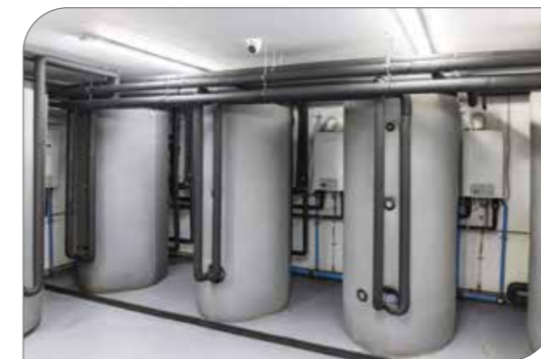
Domestic hot water tanks, Fondital condensing gas boilers.
